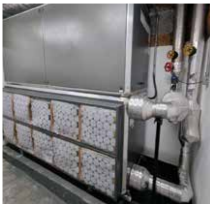
Novo fan coil
