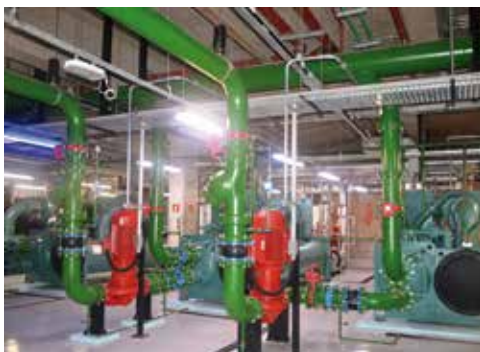
CAG com chillers York
